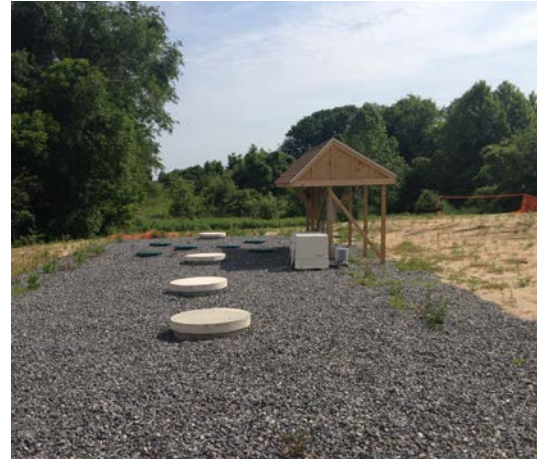
10,000 gallon system servicing a retail development
